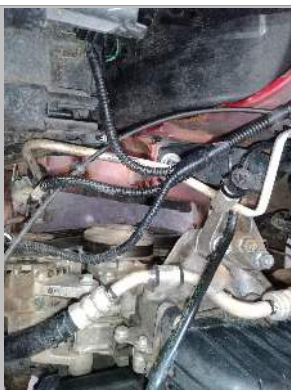
Air conditioner pipes
