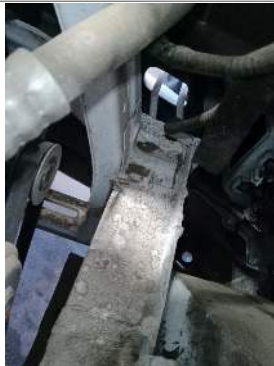
Main Beam Right
