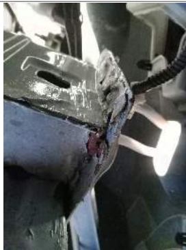
Main Beam Right
