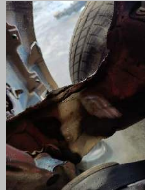
Main Beam Right
