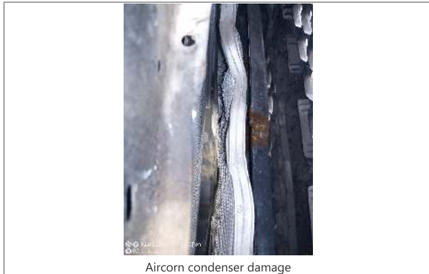
Aircon condenser damage
