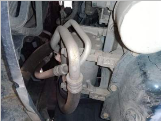
Air conditioner pipes
