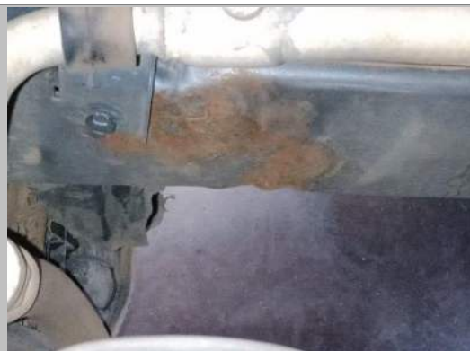
Main Beam Right
