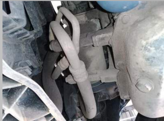
Air conditioner pipes
