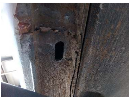
Sill Panel Left
