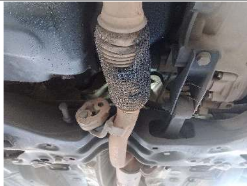
Engine to silencer pipe
