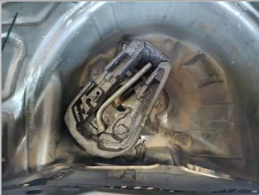
Sparewheel well damaged
