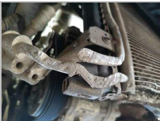
Air conditioner pipes
