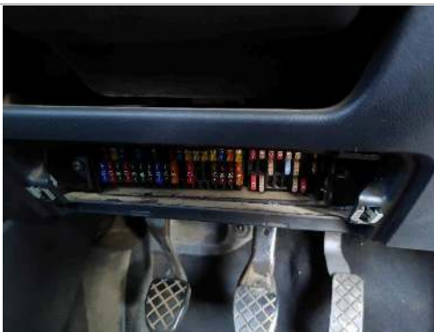
Fuse box and fuses
